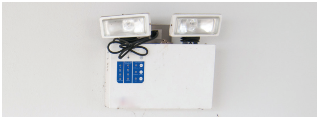
Emergency Lighting Illuminating an Exit Corridor
